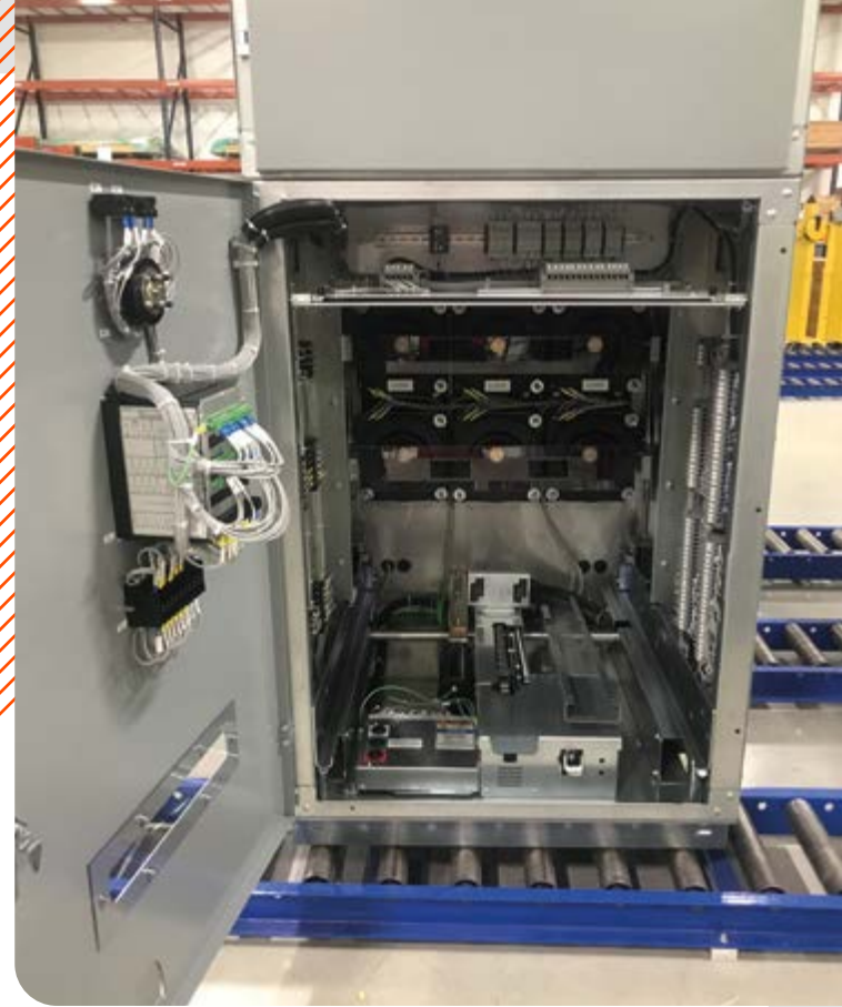
The switch gears assembled at the new JST facility in Florida are engineered-to-order products with a lot of variation from job to job.
