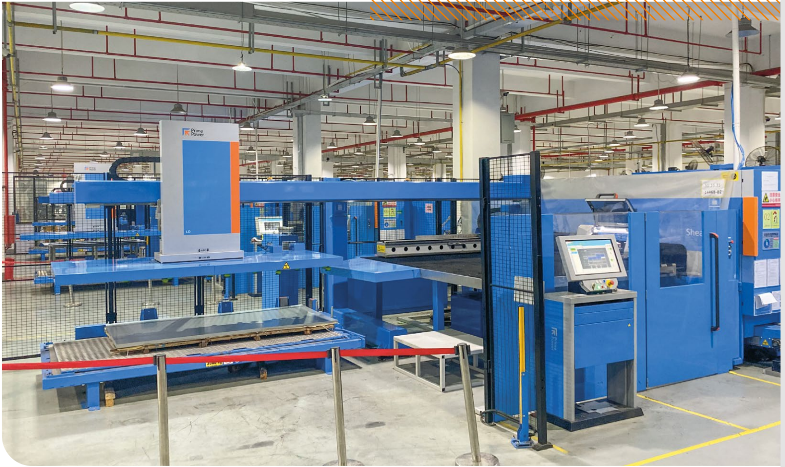
Further to the PSBB line, in SUNSEA AIoT plant 3 Shear Genius SG 1530 machines and 5 eP 1030 press brakes are installed.
