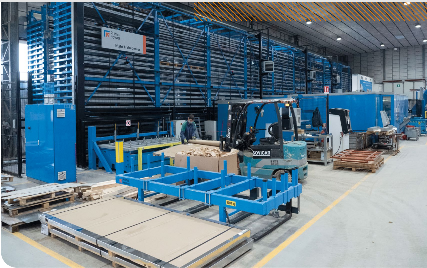
The Night Train automatic storage is connected to the combined Shear Genius and the robotic bending cell, consisting of a Fast Bend panel bender and an eP 1030 press brake.
