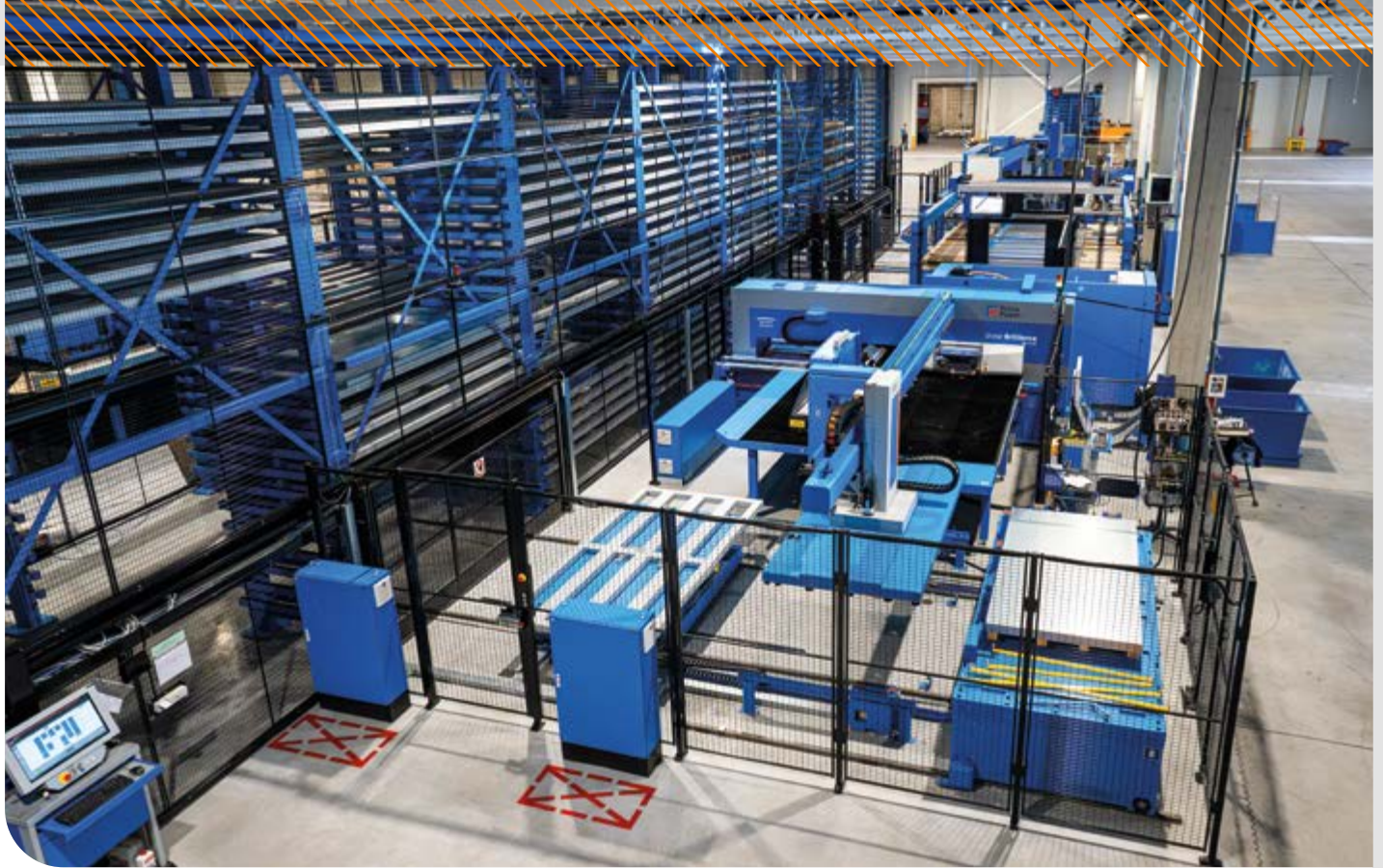
The FMS system installed at Stansefabrikken includes the PSBB line and the automated Night Train warehouse, which allow for automatic, continuous material and data flow.
