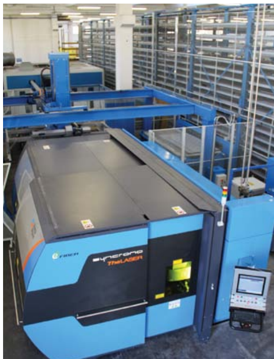
The Sincrono Fiber installed at Rizzato is connected to the automated and synchronized Night Train Material Management System (MMS), which allows a 24-hours-a-day operation for processing continuity.
